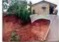
IN DANGER: A cut slope near the government veterinary hospital at Sanoor near Karkala collapsed on Thursday
